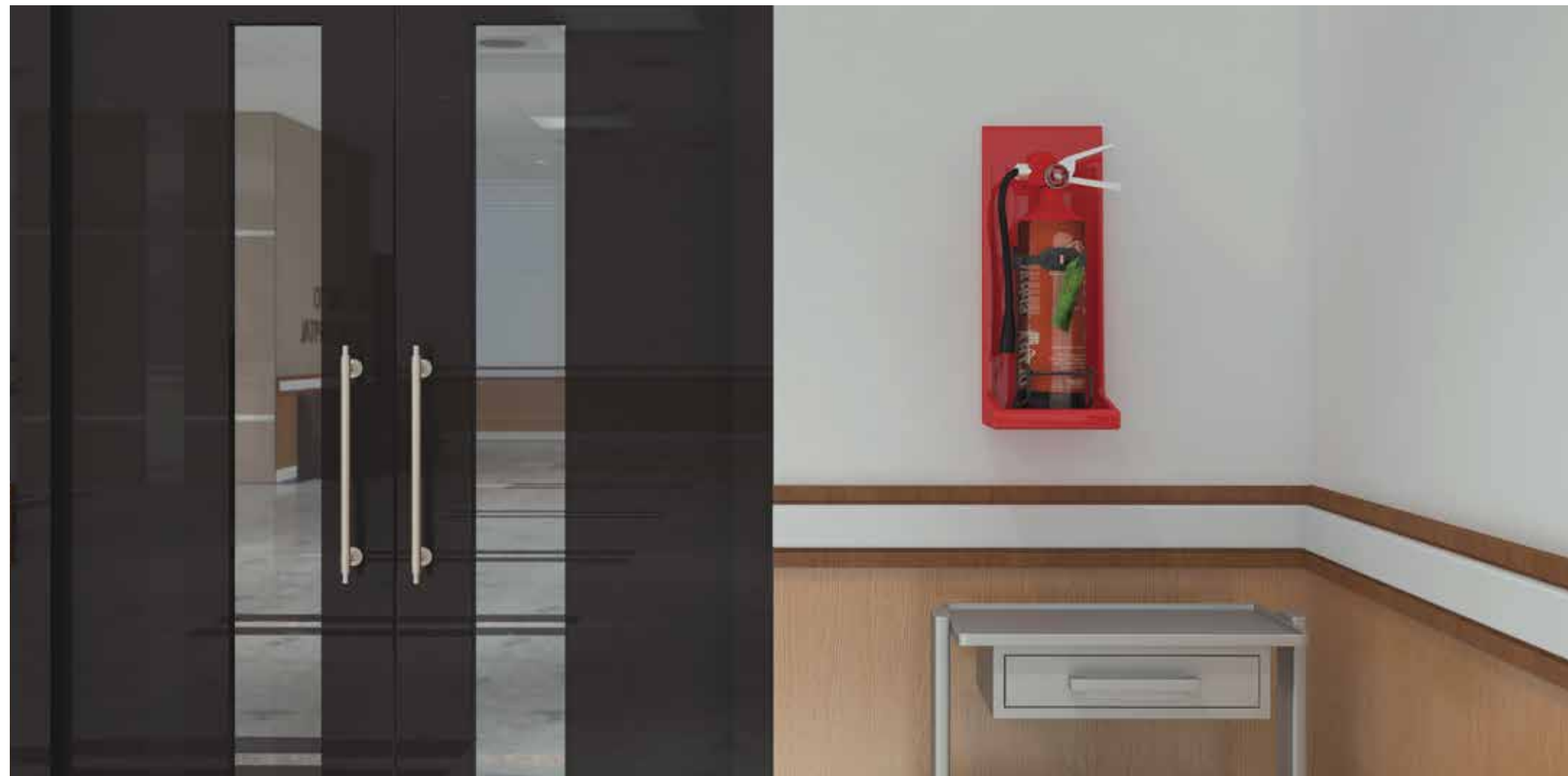
FIRE FIGHTING SYSTEM
